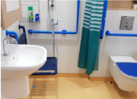
Photo 14: Colour contrasted horizontal and vertical grab bars, toilet seat cover, flush handle/button, sink faucet and handrails
