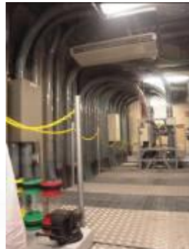
Pneumatic tube interchange
