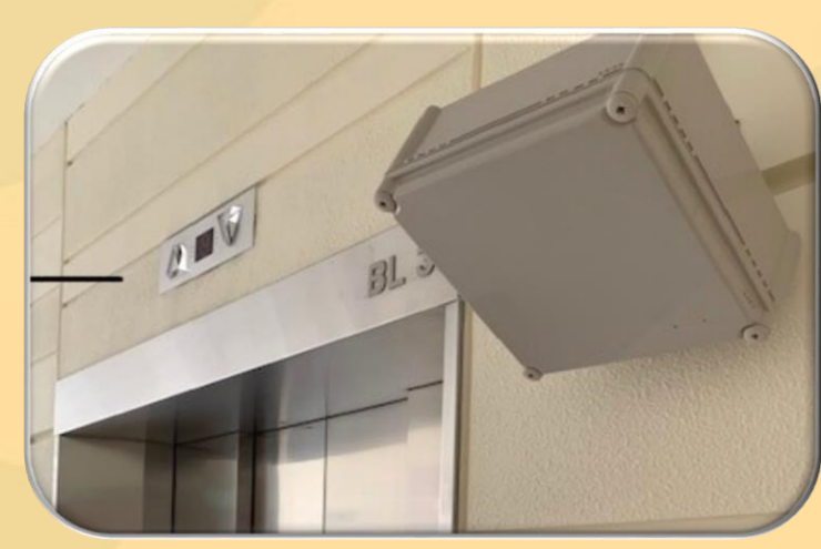
RFID reader at the lift lobby (e.g. non-permitted area)
